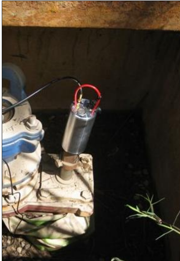
Figure 25 the 'A' Sensor attached to a valve spindle
